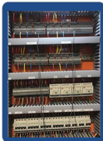
Power Distribution Industrial Panel
