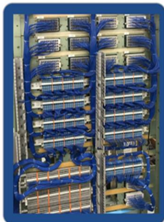
Railway Signalling Panel
